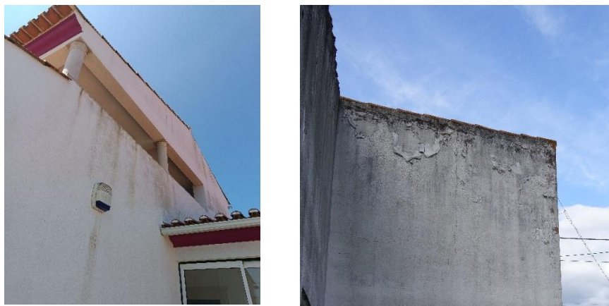
Fig. 3 (left) and Fig. 4 (right) showing the impact of moisture damage and associated biological colonisation on poorly resolved and protected verges and parapets.
